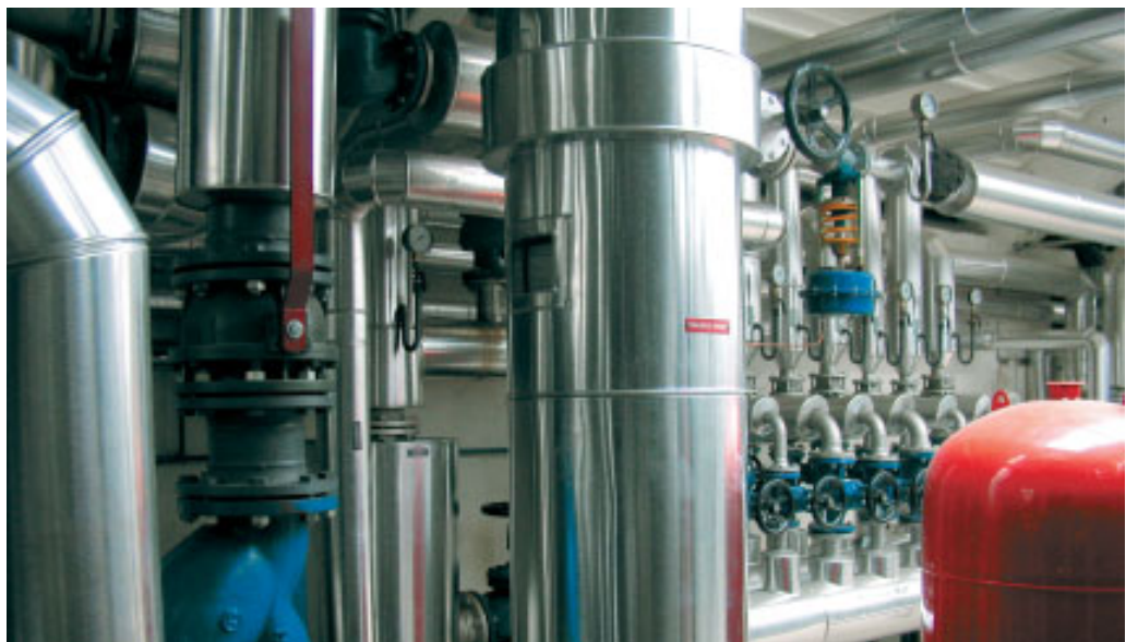
Kotlovnica v Fructalu
